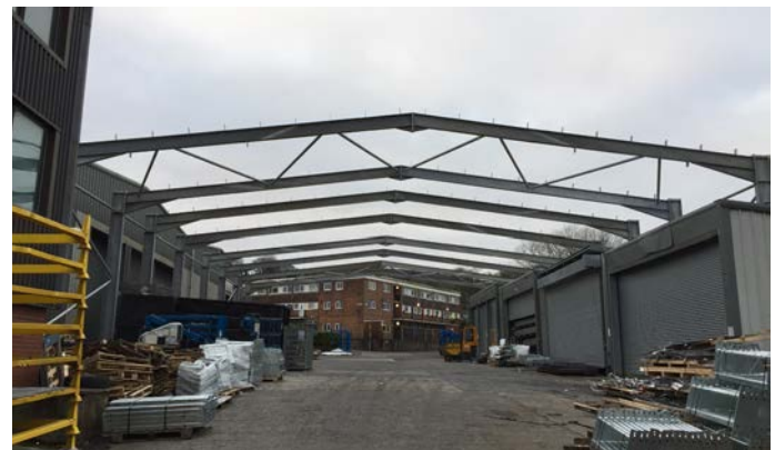
Construction of the new roof for our Laser Yard started in December 2018
